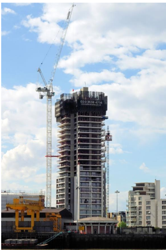
The precast balconies being incorporated into the frame's construction, with the precast cladding panels following below. Image: Marble Mosaic.
