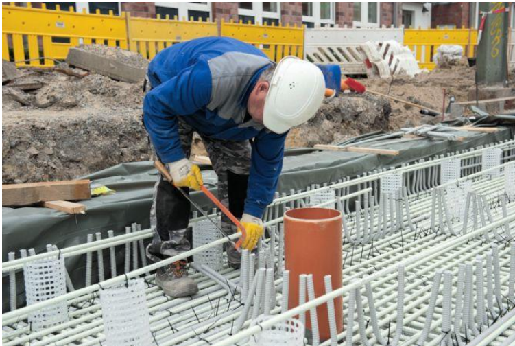
ComBAR reinforcement bars are cut to size by hand saw Image: Schöck Ltd.
